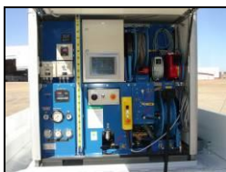
IWU Operator Panel
